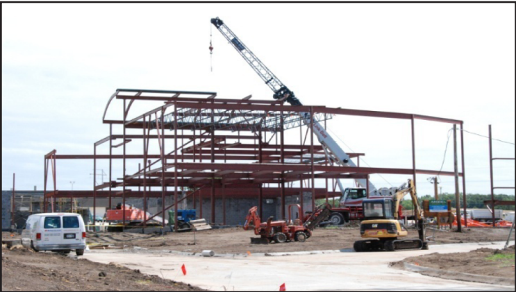
Construction in full swing on the "J. Paul and Eleanor McIntosh College of Nursing" in Norfolk, Nebraska. Scheduled completion date is July 2010.
