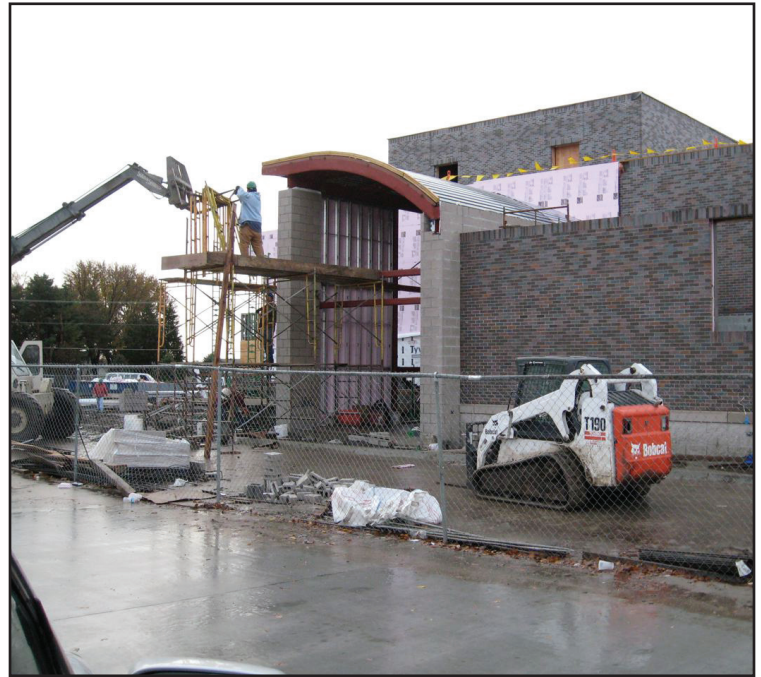
Construction on the J. Paul and Eleanor McIntosh College of Nursing in Norfolk. Photo by Ruth Macnamara 10/30/2009
